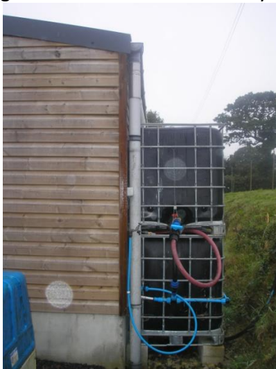
Rainwater harvesting system
