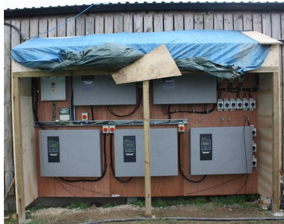
The inverters supplied by ELTEK renewables
